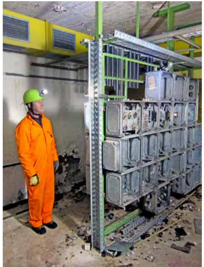
Empty electrical distribution racking with Richard West on guard. Photo Tim Wellburn
